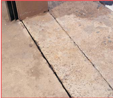
1. Expansion joint and crack to be filled.
